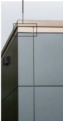
Dummy modules used to cover smallest parts.
